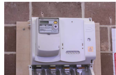
Shown With Meter Fitted
