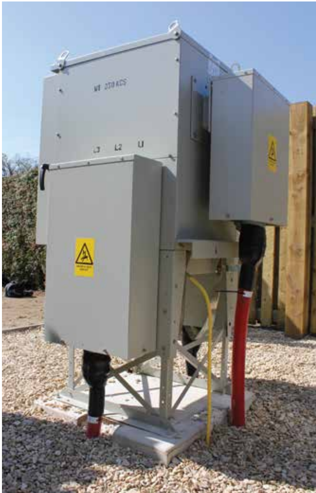
Outdoor free standing with bottom entry cable box
