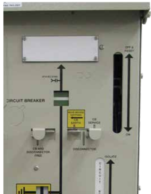
Circuit breaker mechanism
