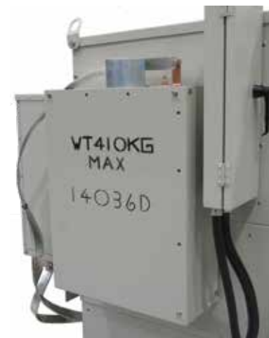
Top entry cable box
